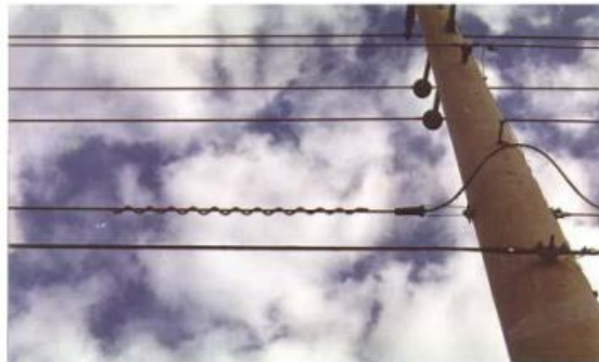
Figure 11: Aeolian Vibration damper installed at the end of a fiber span.
